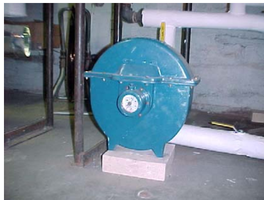
Pictured above is the original Cast Iron "E" size condensate meter with a local mechanical counter.
